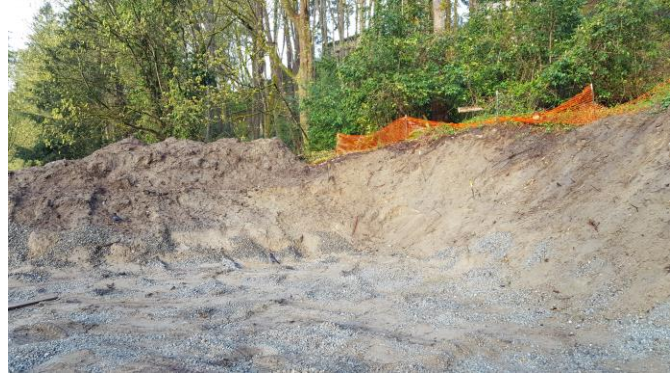
Plate 1. View of temporary excavations at the southwest corner of the building pad on 4/5/2019, looking southwest
